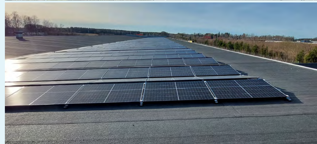
Top picture - Solar panels on our building in Klundert, Netherlands. Bottom picture - Solar panels on our building in Tibro, Sweden.
